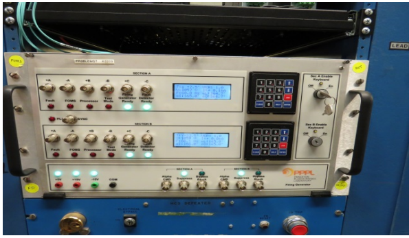
Fig. 15. Firing Generator front panel
