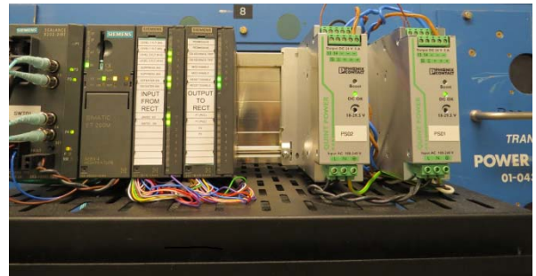
Fig. 19. PLC used in the Tranrex power supply
