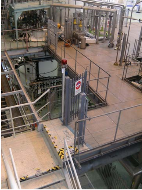
Figure 6. Good safety precautions near magnetic fields.
