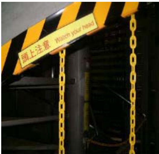
Figure 3. Plastic chains warn workers of the overhead hazard.
