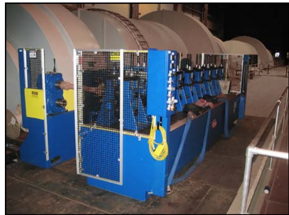
Figure 3. Tube mill for jacketing ITER toroidal-field conductor (installed in the PPPL C-site MG area).
