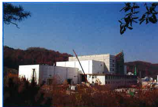
Figure 3. The Korean Superconducting Tokamak Advance Research facility under construction in Taejeon, South Korea.
