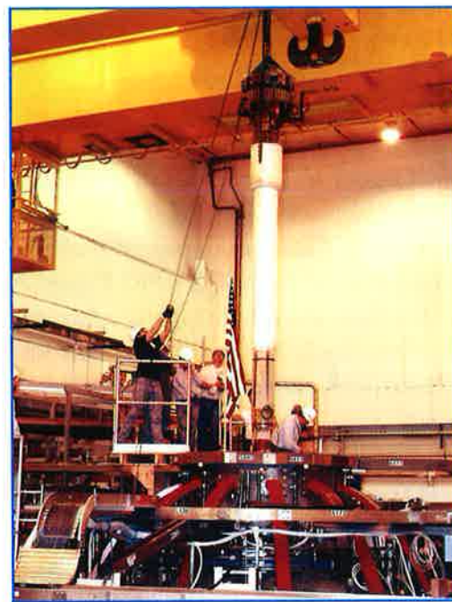
Figure 2. The obmic-heating coil being removed from the center stack of the National Spherical Torus Experiment.
