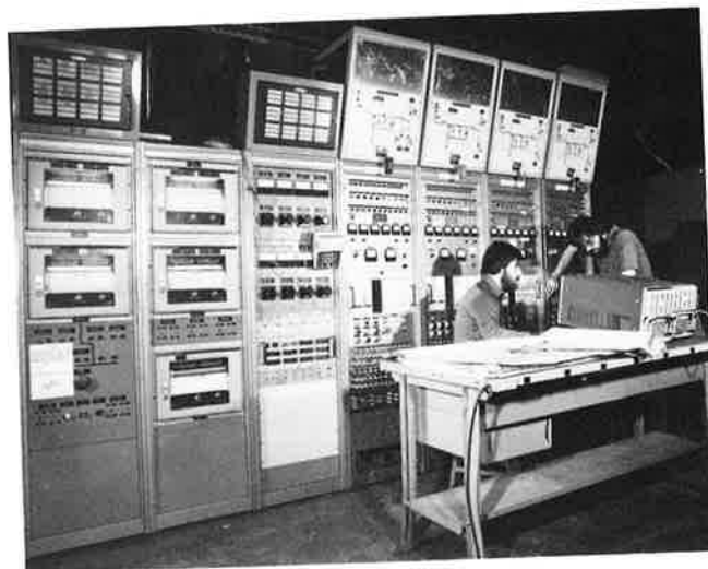
Figure 37. PLT/PDX neutral beam power supply console.
