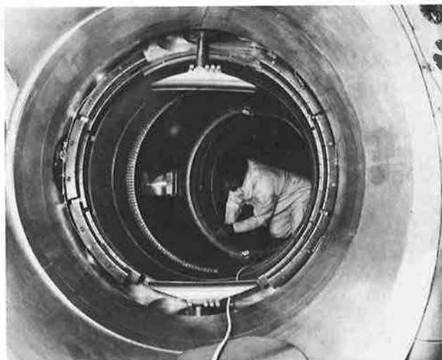
Figure E. ICRF \frac{1}{2} -turn coil installation on PLT.
