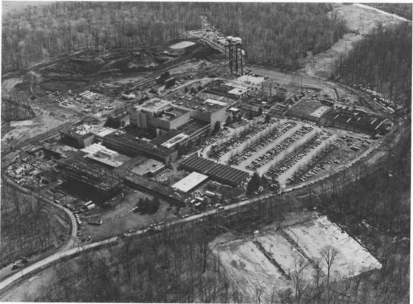
Figure 37. Current construction at C-site, Plasma Physics Laboratory. TFTR site is at upper left.
