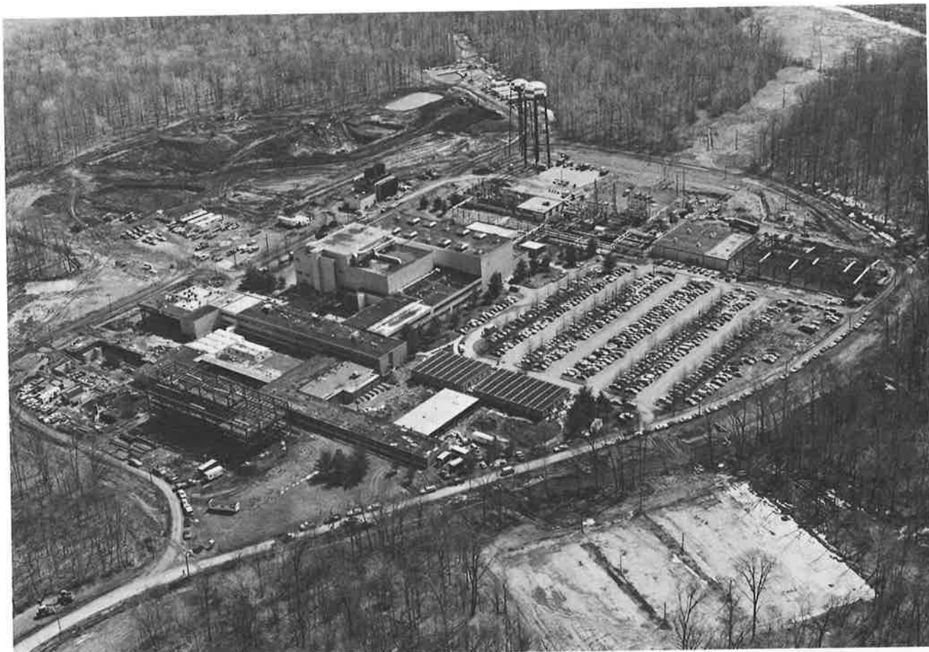
Figure H. Construction at C-site, Plasma Physics Laboratory. TFTR site is at upper left.
