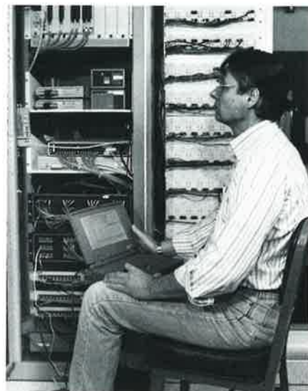
A computer technician troubleshoots PPPL's Network infrastructure.
